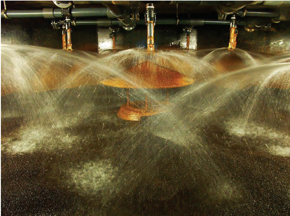
Figure 2: Full-scale trickling filter at Oasen WTP Lekkerkerk. Raw water is sprayed directly on top of the filter bed. The central outlet with cone is used for drainage of backwash water.
