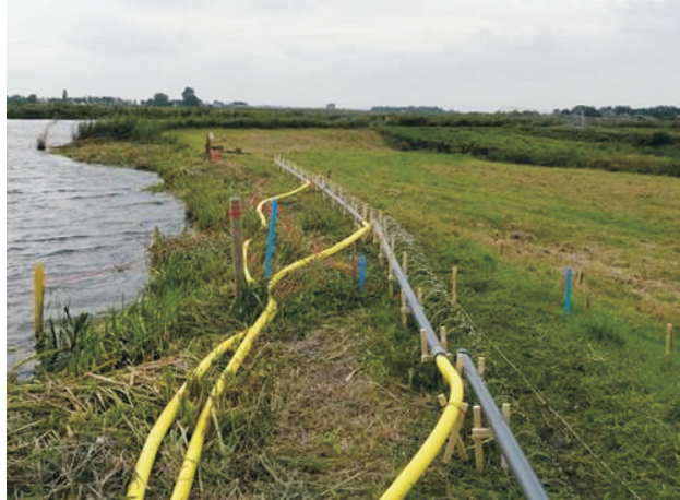
Figure 2.7: Wetting system placed at the crest of the dyke
