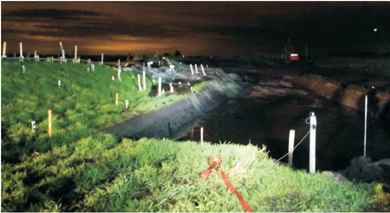
Figure 2.9: The moment of the failure of the dyke at the Leendert de Boerspolder in correspondence of Section Centre and Section South
