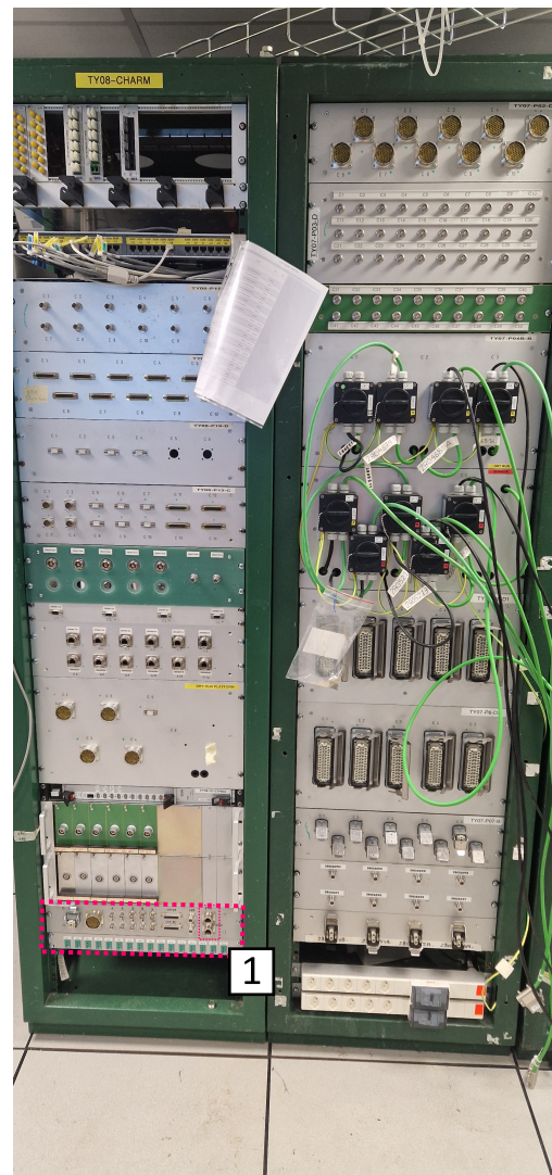
Figure 4.9: Patch panel in the mock-up room. 1) The connectors for the overhead conveyor, with on the right two Ethernet connectors.
