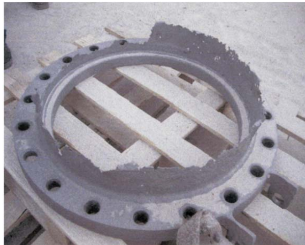
Figure 19: Break within the ESWS (IAEA, limited distribution b)
