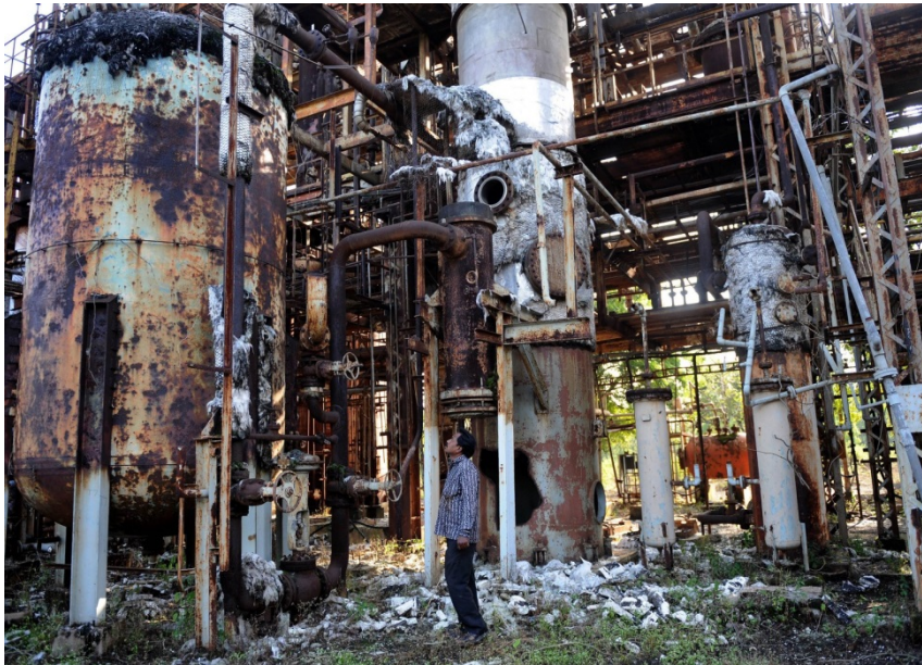
Figure 16: Bhopal chemical plant (Anderson, 2018)
