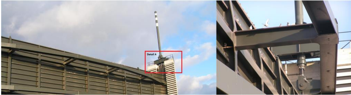
Figure 7 Hydraulic cylinder on the vertical lifting gate of the Kromme Nol. Left an overview of the total gate indicating detail A which is presented in the right figure. It shows how the piston is connected to the gate.
