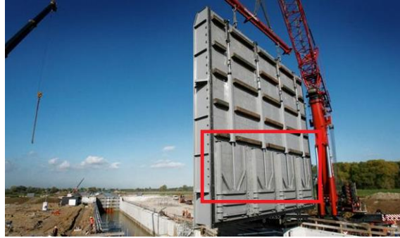
Figure 4 Fill and empty valves in the sluice Empel. The smaller gates are opened and closed in vertical direction by hydraulic cylinders installed on top of the gates. (van Reeken & Rijkswaterstaat, 2014)
