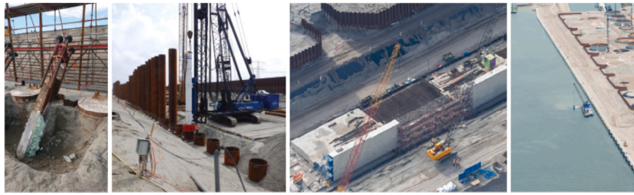
Fig. 2. Construction of the quay wall (a) installation of the MV anchors; (b) installation of the tubular piles in the combined wall; (c) casting of the superstructure segments; (d) dredging.
