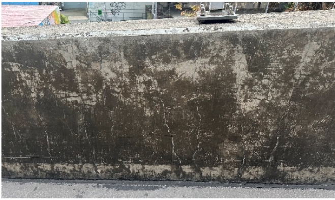
Fig. 1. Early-age cracking causing leakage in water-retaining concrete walls.
