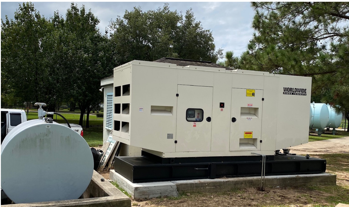
Figure A.3: [Disaster measure] ; Backup Diesel generator. The Backup Diesel generator will provide electricity in the Recovery phase. Depicted is a diesel generator for a water treatment facility in Texas Worldwide Power Products [2023].
