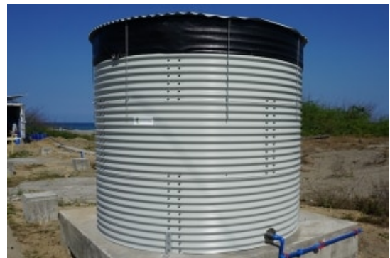
(f) [Salt water-buffer tank] & [Fresh water-buffer tank] are buffer tanks of concrete, build as a basin to ensure stable pressure in the system. The saltwater tank is elevated to ensure constant pressure. The freshwater tank is a location in which the produced fresh water is stored. This ensures pressure in the system and helps the availability of freshwater for the users.
