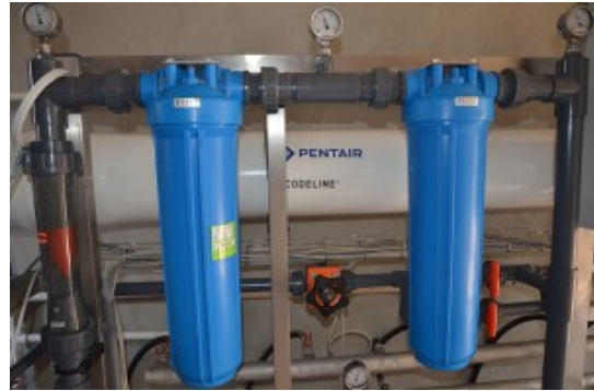
(b) [Pre-filtration] will prevent larger polluting particles to enter the RO, which is an easily clogged membrane. To avoid frequent membrane replacement, the pre-treatment will be designed for your site-specific situation. This can involve sand filtration, cartridge filtration, and more
