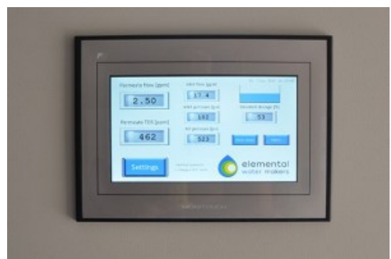
(h) [(Remote) monitoring control] This included all electronics equipment to maintain the system. The units are equipped with internet-based monitoring for remote control and alarm messaging. This is to check in on the water supply from anywhere
