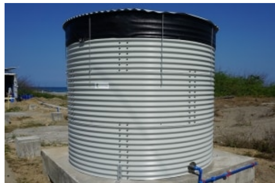
(f) [Salt water-buffer tank] & [Fresh water-buffer tank] are buffer tanks of concrete, build as a basin to ensure stable pressure in the system. The saltwater tank is elevated to ensure constant pressure. The freshwater tank is a location in which the produced fresh water is stored. This ensures pressure in the system and helps the availability of freshwater for the users.
