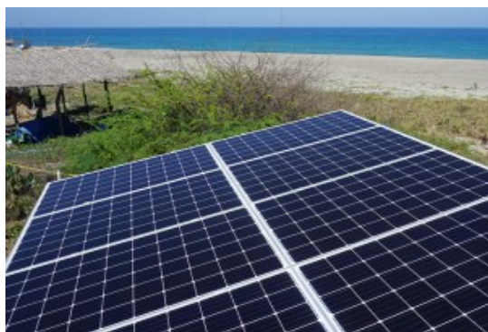
(a) [Solar panels]
