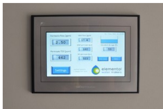
(h) [(Remote) monitoring control] This included all electronics equipment to maintain the system. The units are equipped with internet-based monitoring for remote control and alarm messaging. This is to check in on the water supply from anywhere
