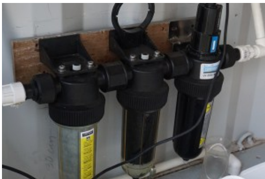
(e) [Post-treatment] is possible specific applications that can add fresh water treatment steps to the system, for example, remineralization, UV treatment before end use, or preservation dosing to make it suitable for longer-term storage.
