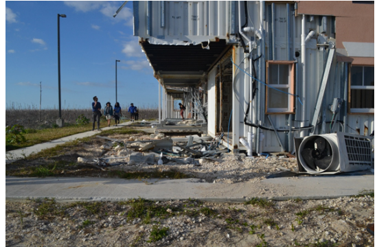
(b) Destroyed dorm on the university campus that had been flooded by a storm surge credit; F. Ortiz
