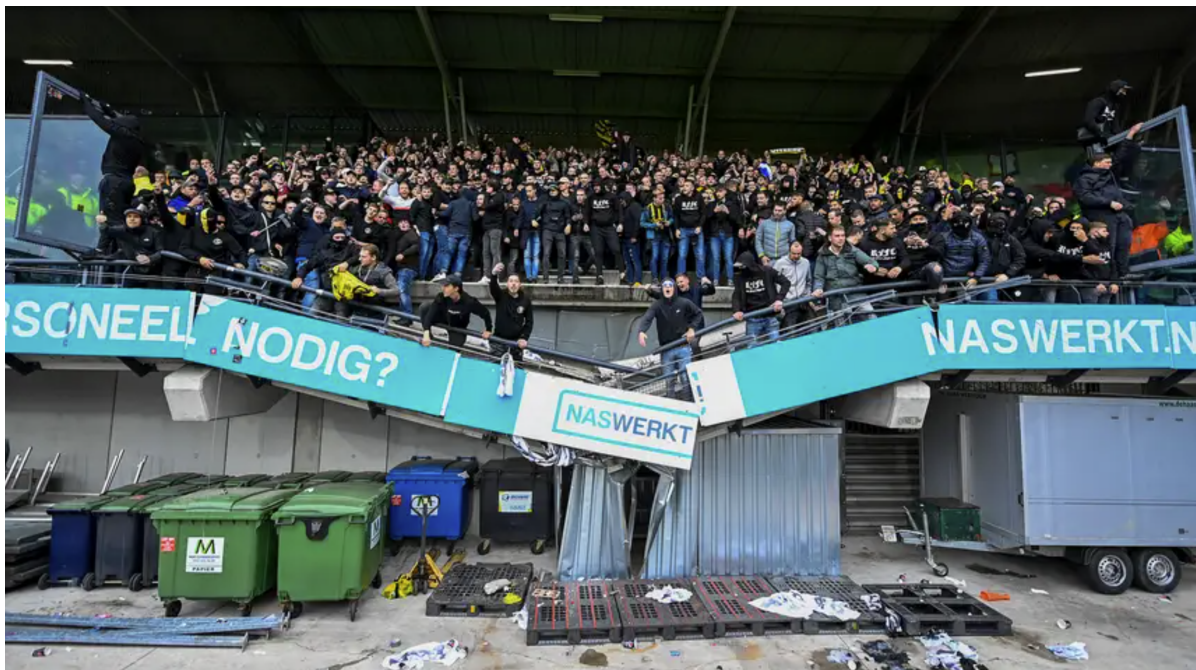
Figure 1.1: The collapsed grandstand element, with people still on top of it. Below the element, the steel container can be seen. Image is taken from NU.nl [1].
