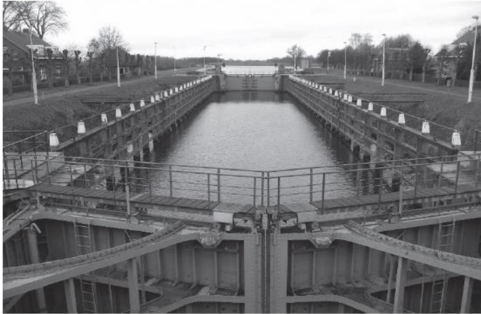
Figure 4-5: Example of Mitre Gate in The Netherlands [22]
