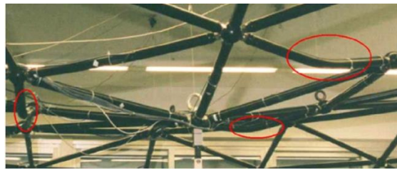
Figure 25: Local member buckling [14].
