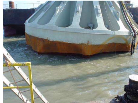
Figure 3.4: Failed attempt during installation at Wilhelmshaven
