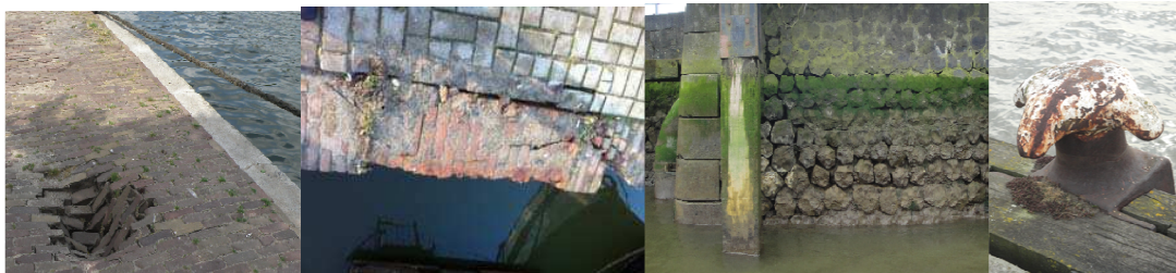
Figure 9 Photographs of damage discovered by a visual inspection (class 1b)
