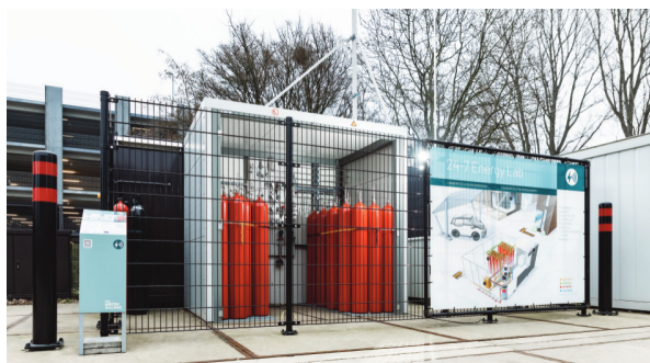
Figure 2.3: The outdoor, fenced compound of the 24/7 Energy Hub pilot at The Green Village. The orange cylinder racks are the high-pressure hydrogen storage tanks; a control/power cabinet stands to the right [27].
