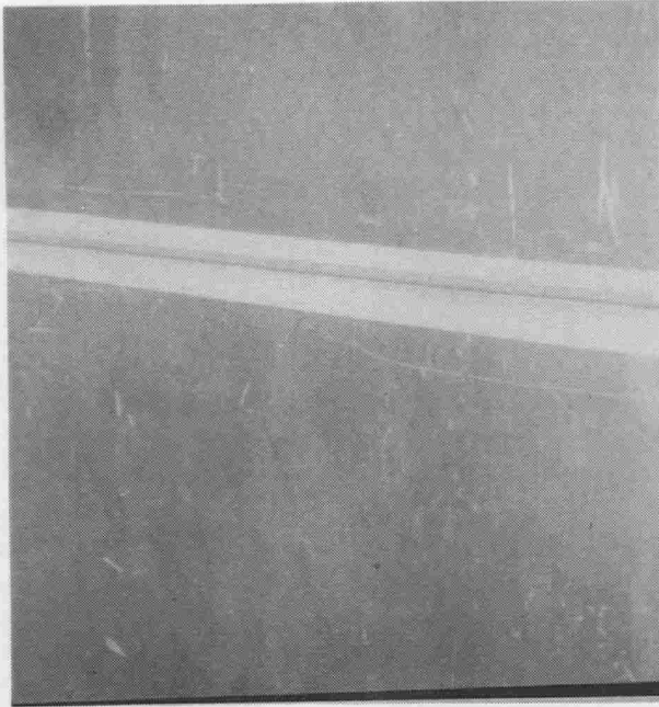
Photo 17. View on the welding joint on the welding side, ready for welding
