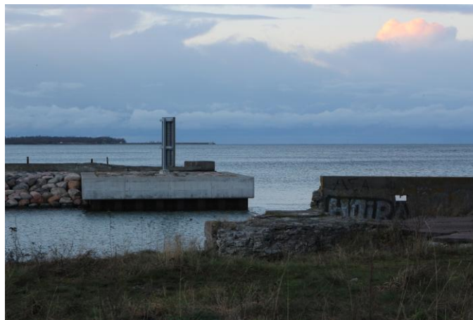
Existing coastal conditions – derelict structures and a 4m drop to water-level.
