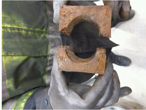
Fig. 5 Corroded and broken nut at Ramspol Barrier. (Image: Courtesy of Rijkswaterstaat, Tycho Busnach.)
