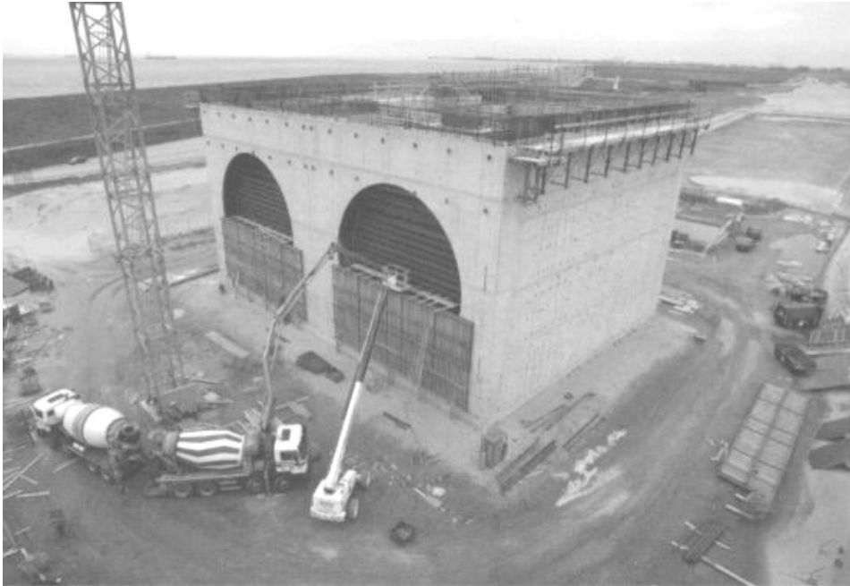
Figure 4-11 Entrance shaft of the Westerschelde tunnel constructed as a caisson at ground level
