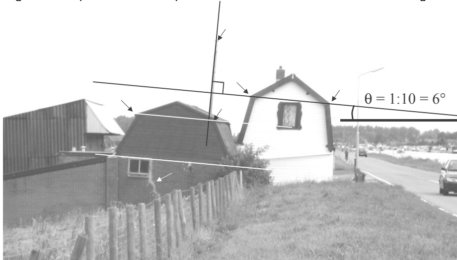
Figure 4-4 Settlement of a house (rotated) due to dewatering a construction pit
