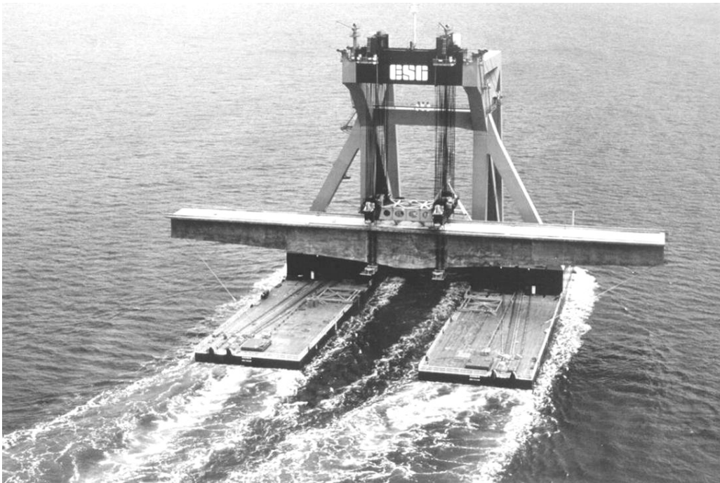
Figure 5-4 Floating crane Svanen (Ballast Nedam) with bridge girder for the Westbridge over the Great Belt, Denmark
