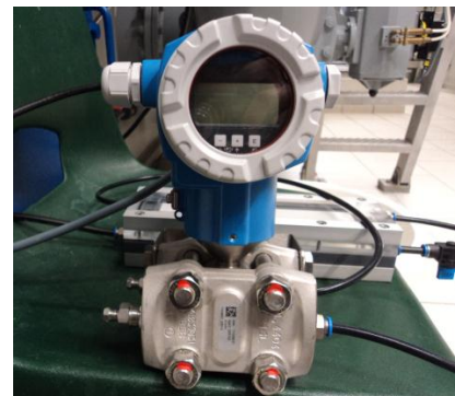
Figure 3-3 - Differential pressure transmitter measuring the feed channel pressure drop
