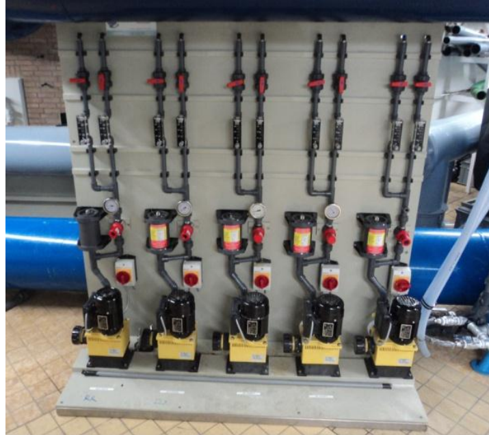
Figure 2-10 - Dosage pumps used for flow control to measuring devices
