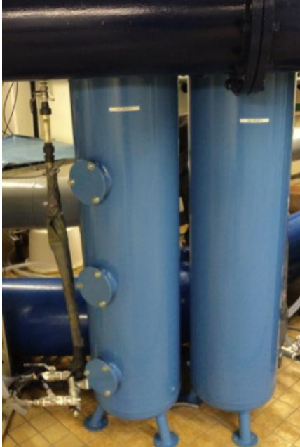
Figure 2-9 - Activated carbon pressure vessels
