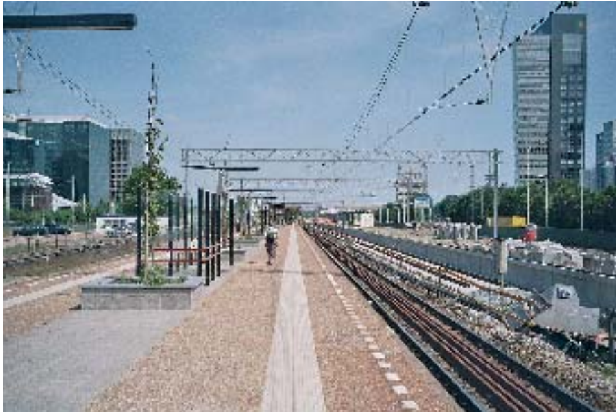
Figure 9.8 A picture of the current Zuid/WTC sta- tion, showing the width of the infrastructure bundle dividing the Zuidas. To the left is the WTC, to the right, the ABN Amro building. A temporary HST platform is being con- structed
