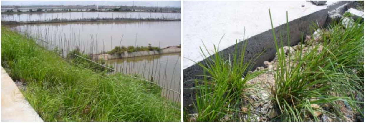
Figure L-16. Types of inner dike slope protection using grass layers and steel sheet piles
