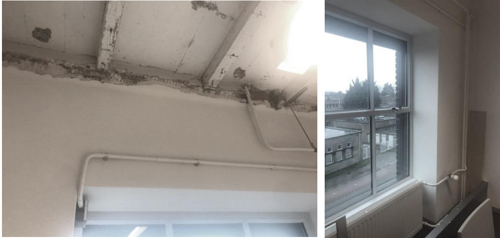
Figure 41 The network of cable conduits and pipes attached to the surface
