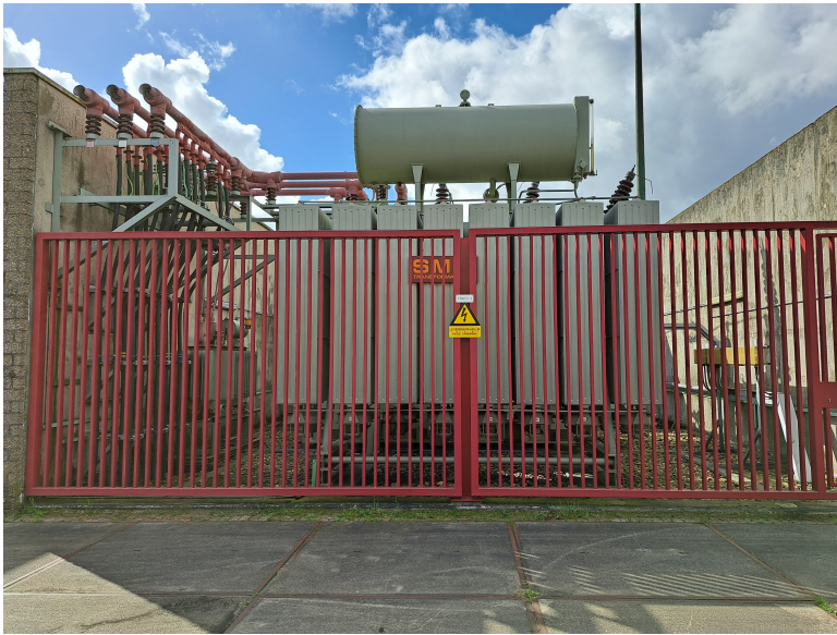
Figure 1.6: The three-phase transformer used as a case study (with permission from Alliander N.V.).
