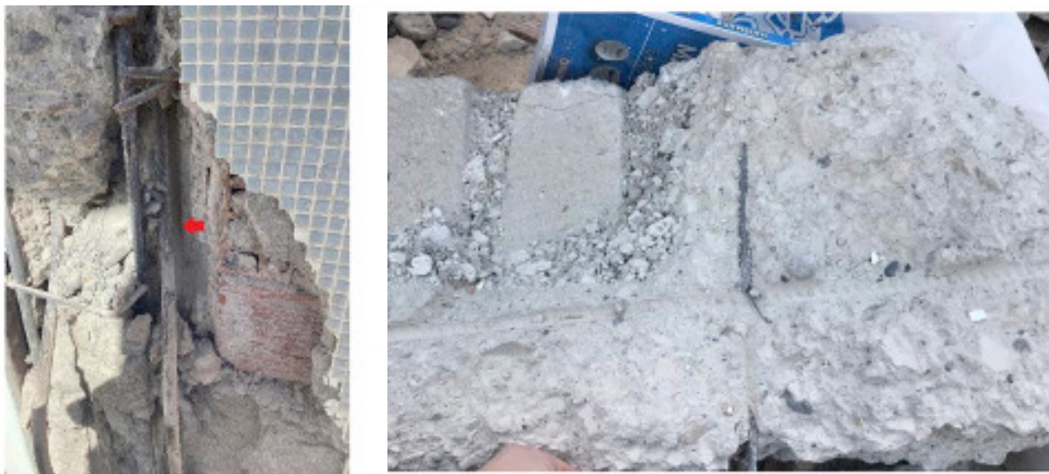
Figure 3.36: Photos from the reconnaissance study depicting rebar related issues in a structure (Sezgin et al., 2024)
