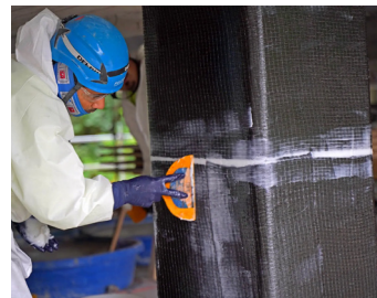
Figure B.10: The application of fibre reinforced polymers to a column (Structural technologies, n.d.)
