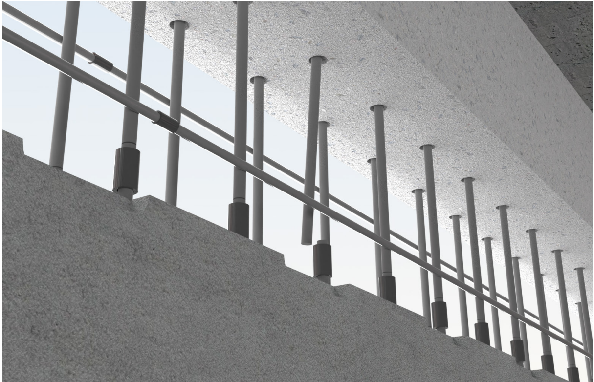
Figure J.15 - Step 15: The last rebars are fastened by sliding them into pre-drilled holes in the ceiling. In order to allow fastening in this relatively narrow space, couplers must temporarily be slid down to allow insertion of the final rebar segments.
