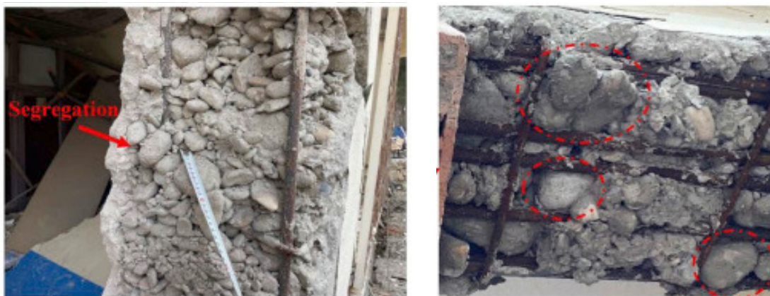
Figure 3.35: Images from the reconnaissance study depicting aggregate related issues in a structure (Sezgin et al., 2024)
