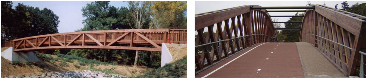
Figure 3.2: Two examples of truss bridges. In the left picture the deck is placed somewhere halfway the top and bottom chords. The right picture shows a timber bridge near Harderwijk where the deck is positioned at the bottom chord. Also noticeable here are the steel cross beams providing lateral stability to the top chord. [7].
