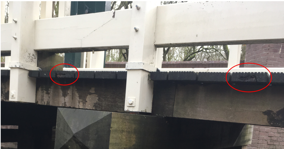
Figure 7.9: End grain surfaces of the deck boards are overall still in good condition. A few boards show beginning amounts of wood rot (highlighted with red circles).
