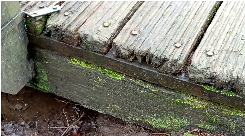
Figure 7.18: End grain surfaces of the deck show large amounts of wood rot.
