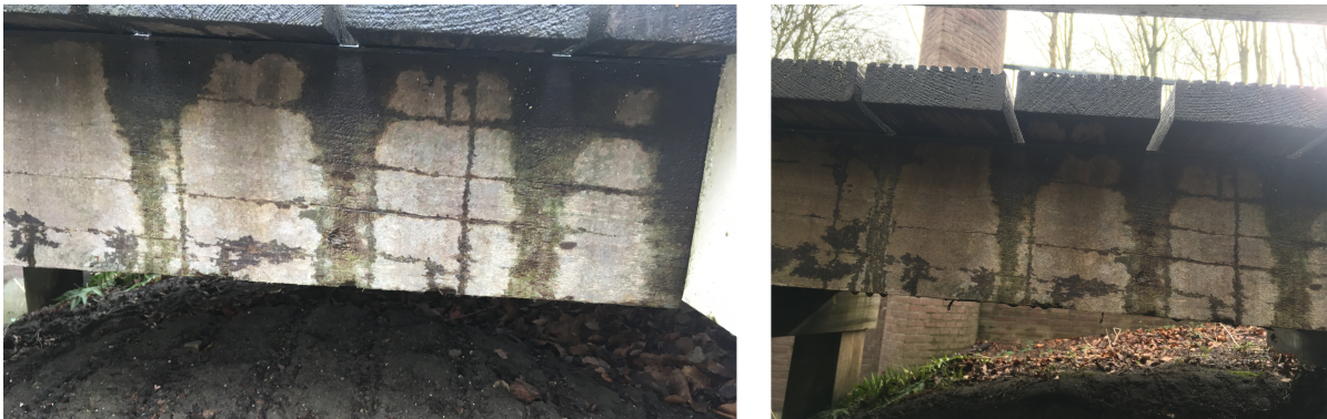
Figure 7.12: Left: Large parts of the railing, covered with a layer of paint, show no visible decay. Right: Longitudinal connection showing paint erosion but no visible sign of decay.
