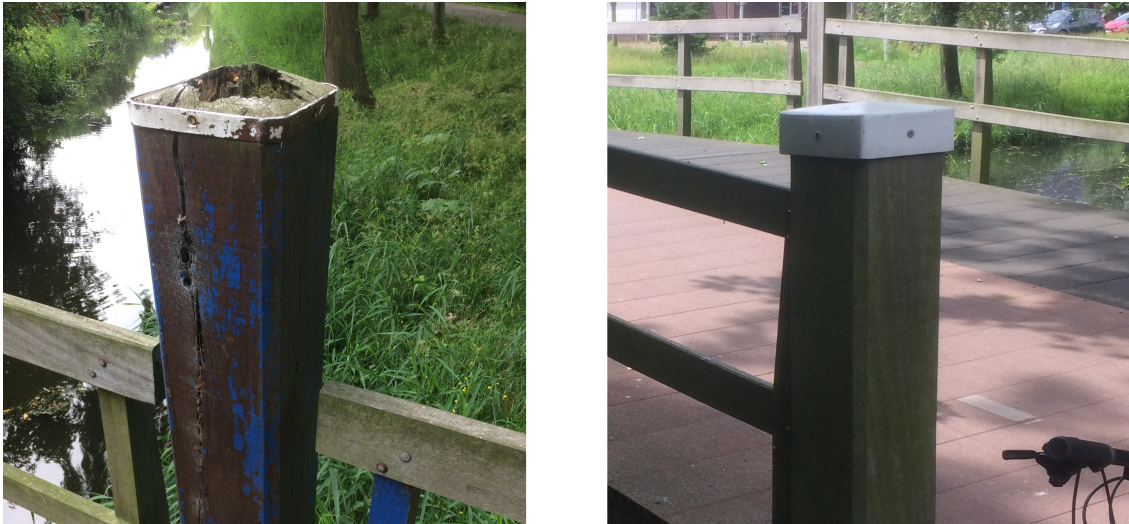
Figure 3.6: Left picture shows an example of a bridge post with unprotected end grain surface. On the right a similar bridge post is shown where the end grain surface is covered to prevent water adsorption. (Both bridges located in Pijnacker)
