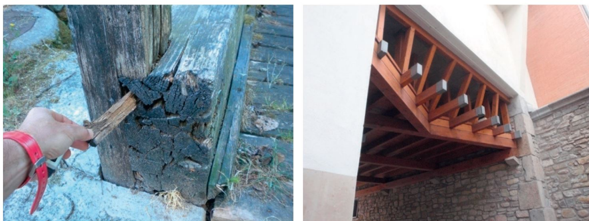
Figure 2.8: End grain protection. Left, timber bridge in Spain without end grain protection of severely decayed main beam. Right, end grain metal covers of projecting exterior beams. [2]
