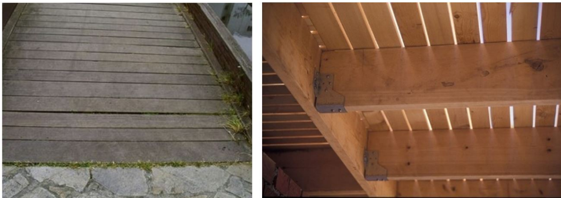
Figure 2.12: Protection from water accumulation. Left, decking with no correct design due to contact board to board. Right, decking well designed thanks to a good separation between boards that avoid water accumulations. [2]
