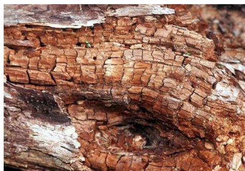
Figure 2.5: Typical example of wood degraded by brown rot [1]
