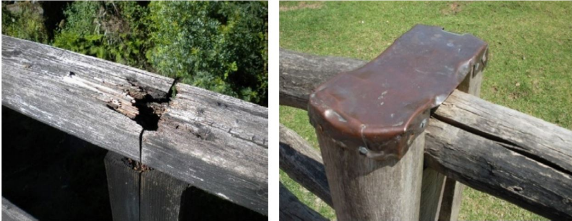
Figure 2.13: Effect of covers. Left, end grain joint on railing without cover protection. Right, fence post with traditional copper cover to protect joint area. [2]
