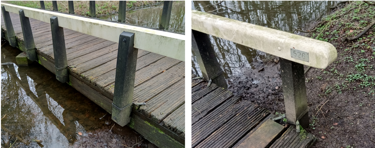
Figure 7.19: The railing, covered with a layer of paint, shows no visible decay.
