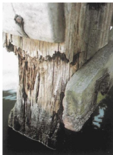
(b) Soft rot and its eroding effect [5].
