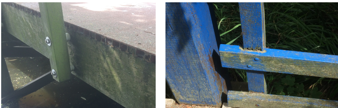
Figure 3.7: Left, railing joint usign spacers to create a gap between the railing post and main beam for drainage and ventilation. Right, railing joint susceptible for water trapping. (Both bridges located in Pijnacker)
