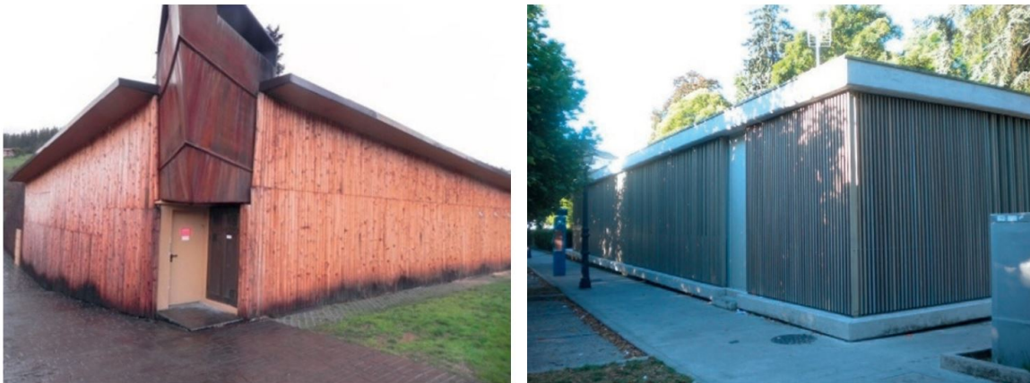
Figure 2.14: Protection from splash water. Left, wetting of cladding made from thermally modified wood in north Spain due to splash water — growth of moulds and disfiguring fungi. Right, cladding in north Spain with correct detail design to avoid splash water. [2]
