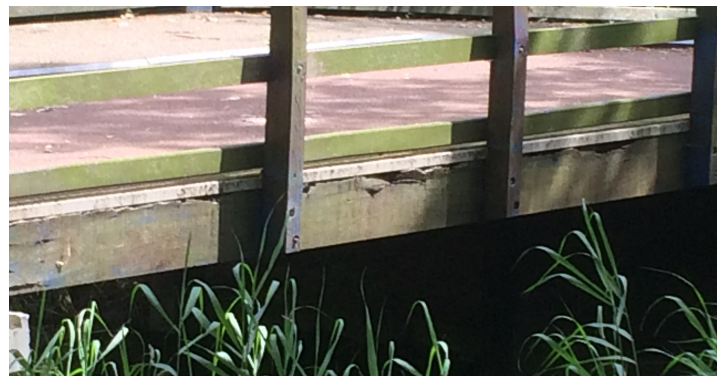
Figure C.3: Example of a timber longitudinal beam suffering from wood rot at the top surface.
