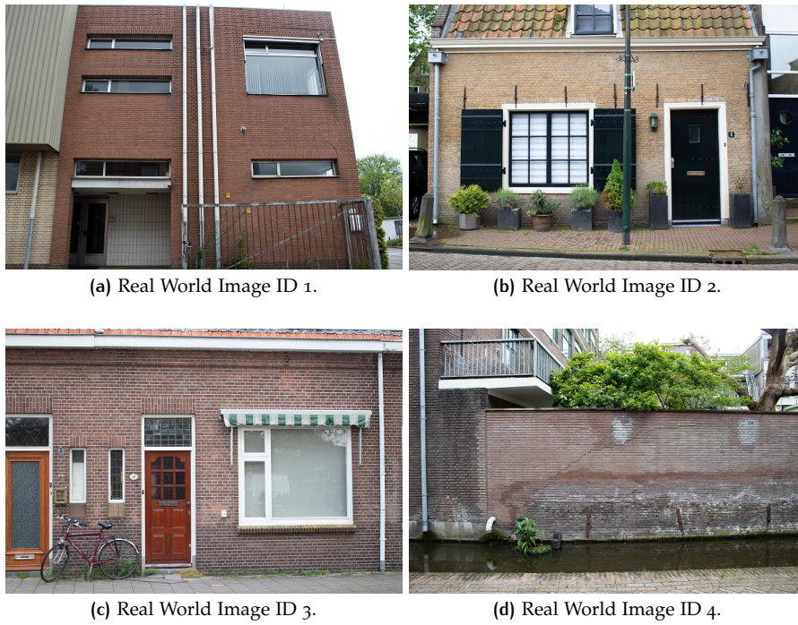
Figure 3.2: Real-world masonry crack patterns obtained from Gouda, The Netherlands.
