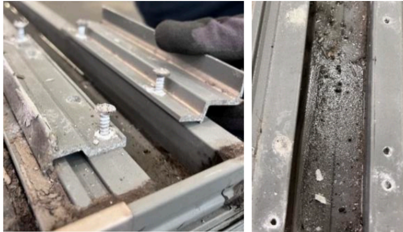
Figure 43: Corrosion of bolts (left) and debris (right) during disassembly experiment of CitiBank unit, conducted by Scheldebouw (image by Scheldebouw).
