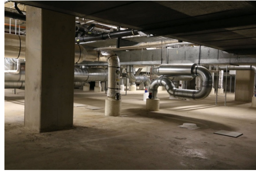
Figure 8: Left: partial cross section of the AMC showing the sub-floors and an inner street. Source: own work based on drawing from Anatomy of the AMC (TU Delft) Right: one of the technical sub-floors. Source: Own picture, 12 July 2018
