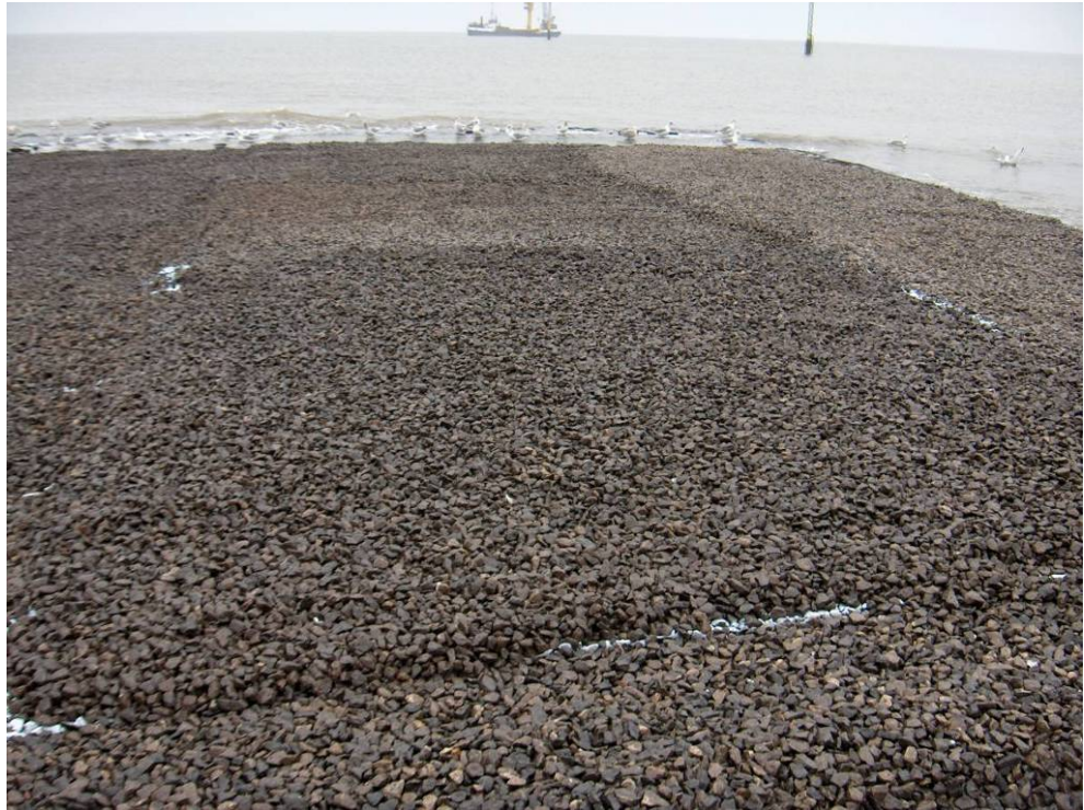
Problem area B: extra 10 cm on top of bad area where stones were too hot.
