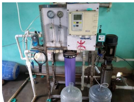
Figure 7.4: Apparatus used for filtering groundwater installed in one of the bottling companies in Tihuria.
