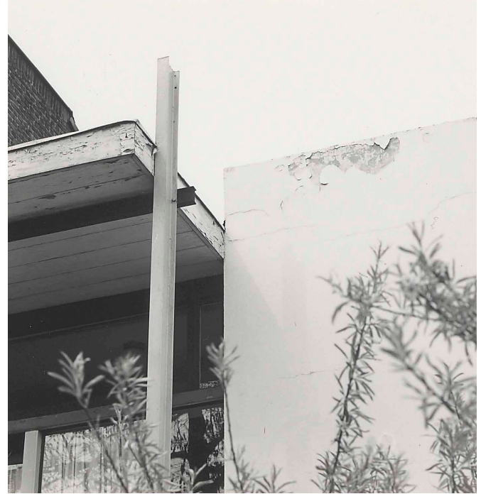
FIG. 1.3 Plasterwork and wood exhibited serious blemishes
