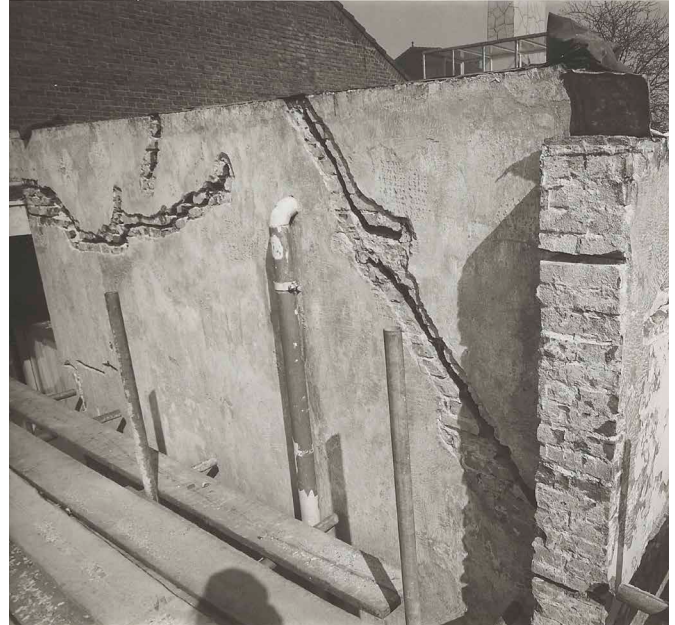
FIG. 1.9 The brickwork displayed deep cracks
