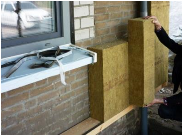
Fig. 2. Placement of outside insulation on the Passive House renovation Nieuwkuijk project by KOW Architecten.
