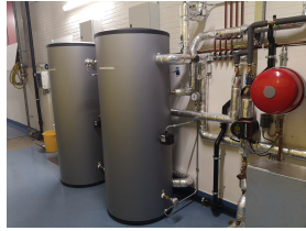
(b) Two 500L water tanks.
