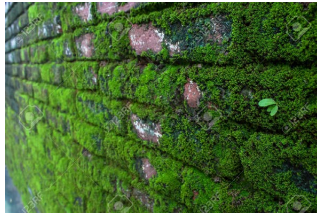
Fig 1.4a: Natural moss growth on walls (retrieved from internet)
