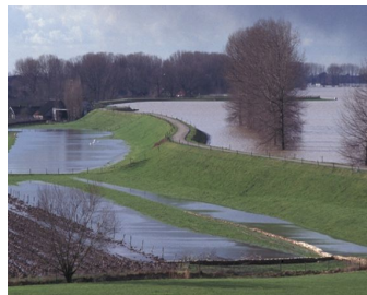
Figure 5.1: Landside ponding due to seepage through a river levee (source: Rijkswaterstaat)
