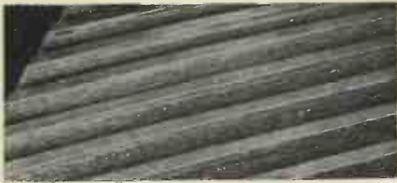
FIG. 6.—SHOWING PITTING BELOW PITCH LINE ON MAIN WHEEL (FORWARD END, AFTER HELIX)
