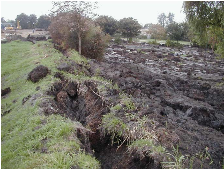
Figure 2.5: End of slipped part of dike (photo by Ir. J.P. Oostveen )
