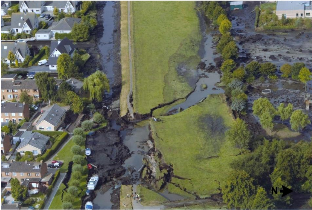
Figure 2.2: Aerial photograph of the breach – north to the right (photo from Utrechts Nieuwsblad)
