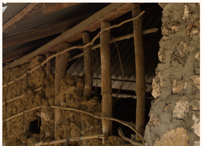
Figure 9: Holes in walls of a house in Watamu
