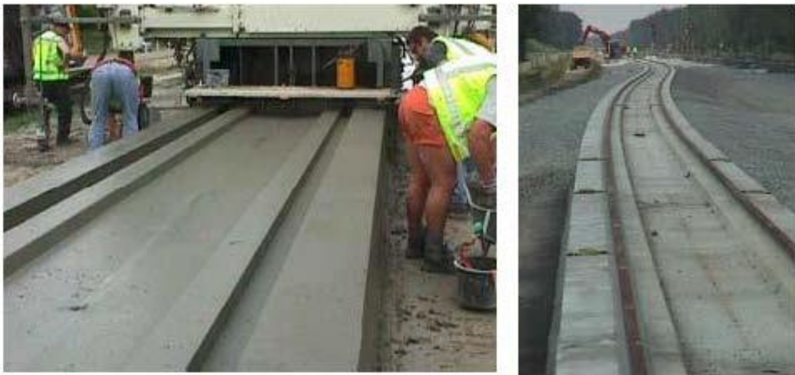
Figure 2 Construction of Embedded Rail with paver (Test track near Best, the Netherlands; source: Strukton Railinfra)
