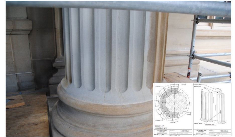
Figure 26. Fluted column repair (patch). Source: The Tradesmen Group
