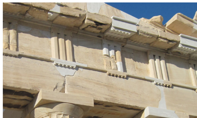
Figure 33. Contrast between old and new marble with visible offset. Source: IIRPS Athens
