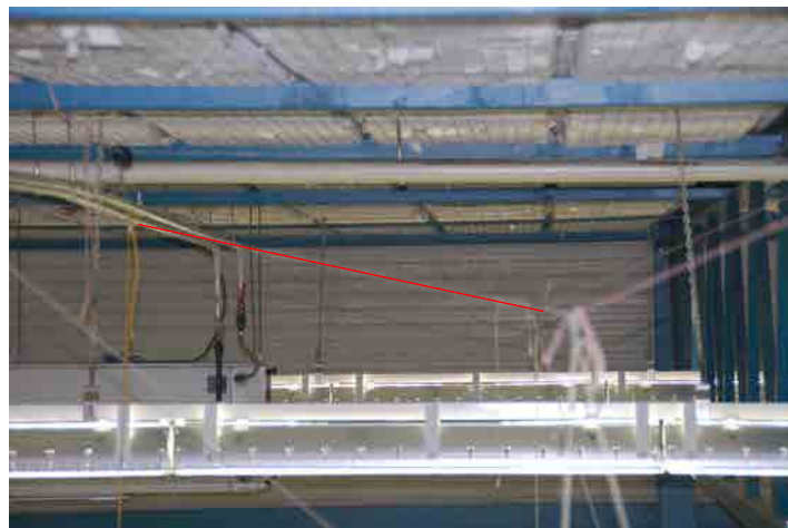
Figure 8-8: Side view of the attachment to the ceiling
