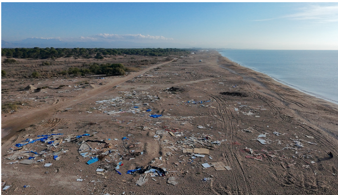
Figure 38. Remainings of Kumköy sheds after demolition, forest and Belek hotel strip at the back. Source: Photograph by the author, January 3, 2025.
