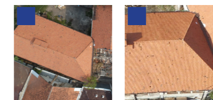
The meeting of the two roofs indicate there was structural or surface issue that needed to be solved, as it is positioned overlapping each other.
