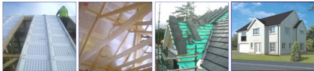
Figure 10: Parietodynamic wall construction. Source: A passive–active dynamic insulation system for all climates (p. 248).
