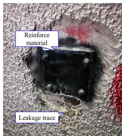
Figure 14. Reinforcement measures in the study site.
