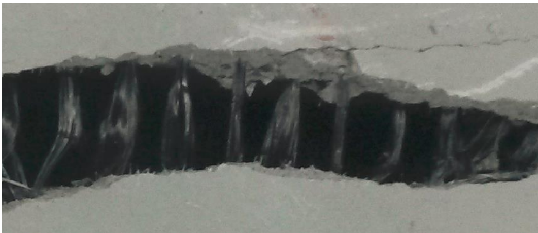
Figure 94: An opened crack in the AC layer with CM threads visible
