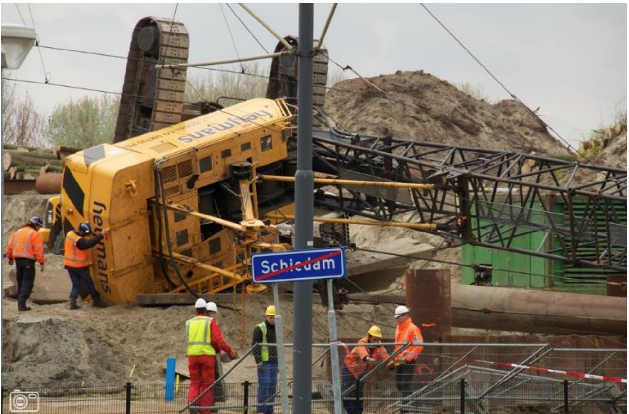
Figure 13: Fallen crane at the A4all project, source: Cobouw
