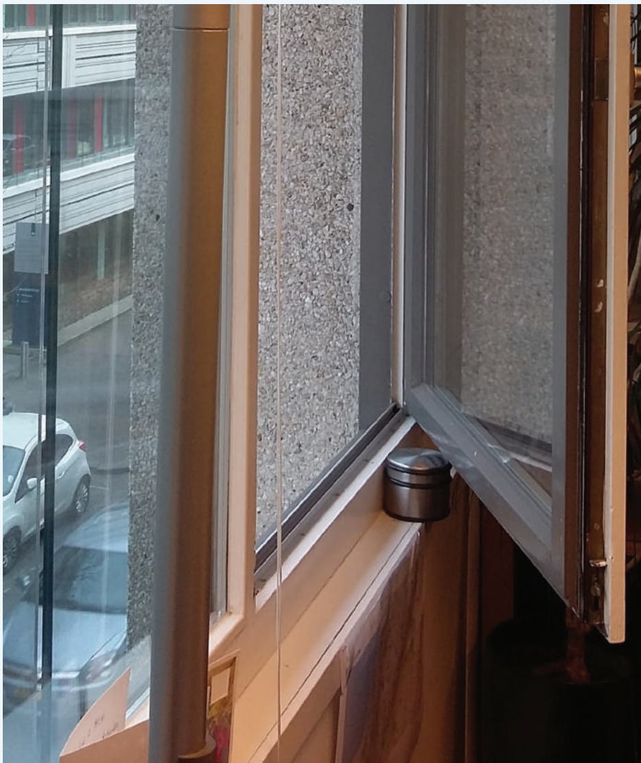
Example of a window with noise ingress
