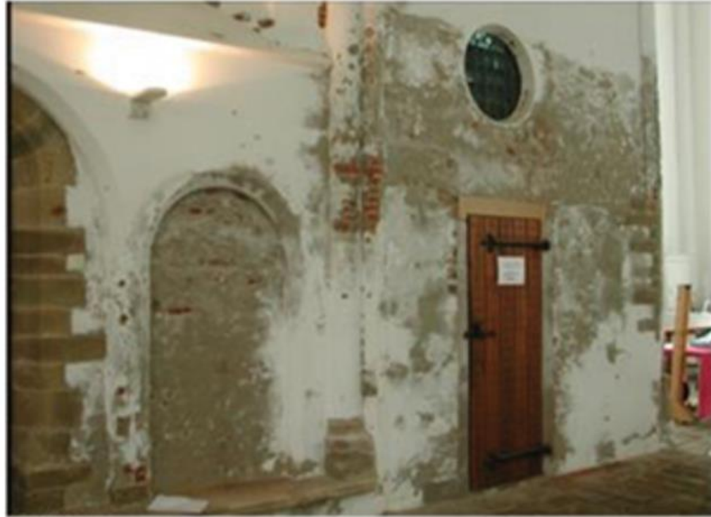
Development of salt crystallization damage over a period of 5 years (Van Hees et al., 2020)
