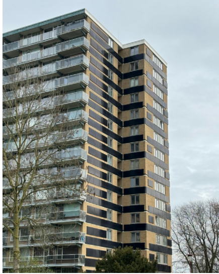
Figure 62: BAPV façade (masonry). Nieuwegein, the Netherlands. Own photo
