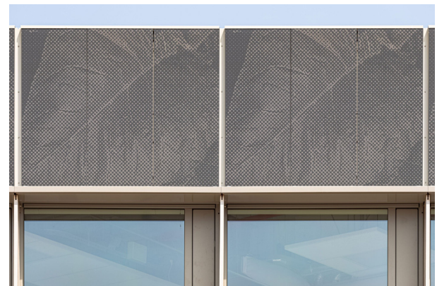
Figure 26: Kameleon Solar: Titaan. Den Haag, Netherlands. Source: De Koning (2024)
